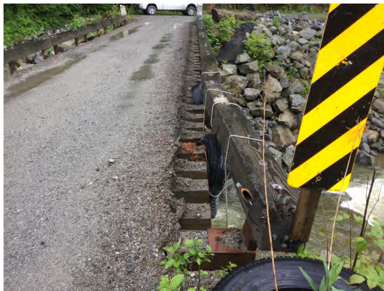
Downstream right bank guardrail has been struck
