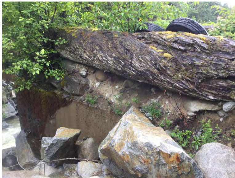
Upstream right bank fender log is largely unsupported behind
