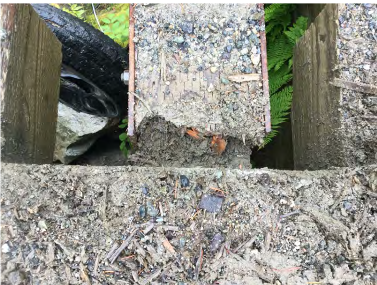
Downstream right bank cross tie damage
