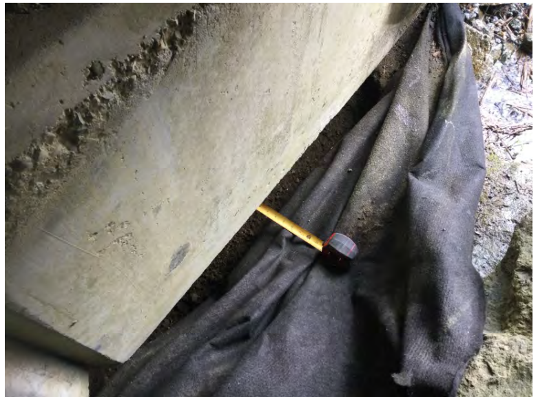
Fill under downstream girder lock block eroded up to 170mm depth behind face x 1100mm width
