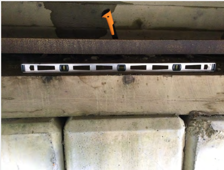
Top of timber sill sloping approximately 20mm downstream over 1200mm length at center of abutment
