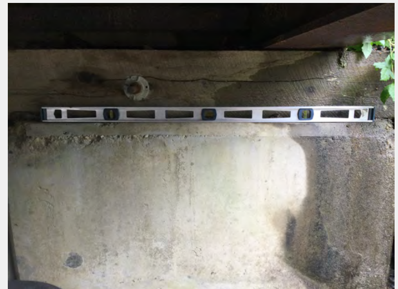
Lock block under downstream girder sloping approximately 40mm downstream over 1200mm length
