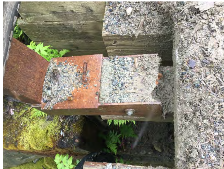
Cross tie damage at downstream right bank
