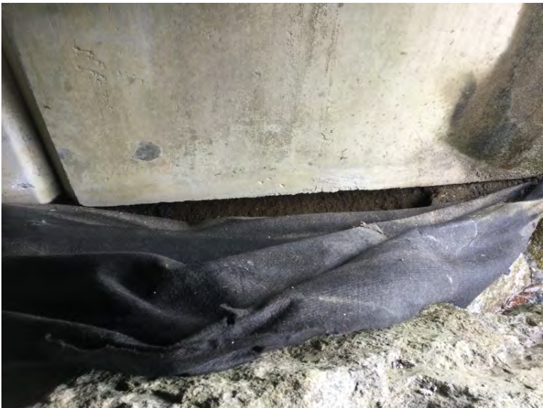
Fill under downstream girder lock block has eroded
