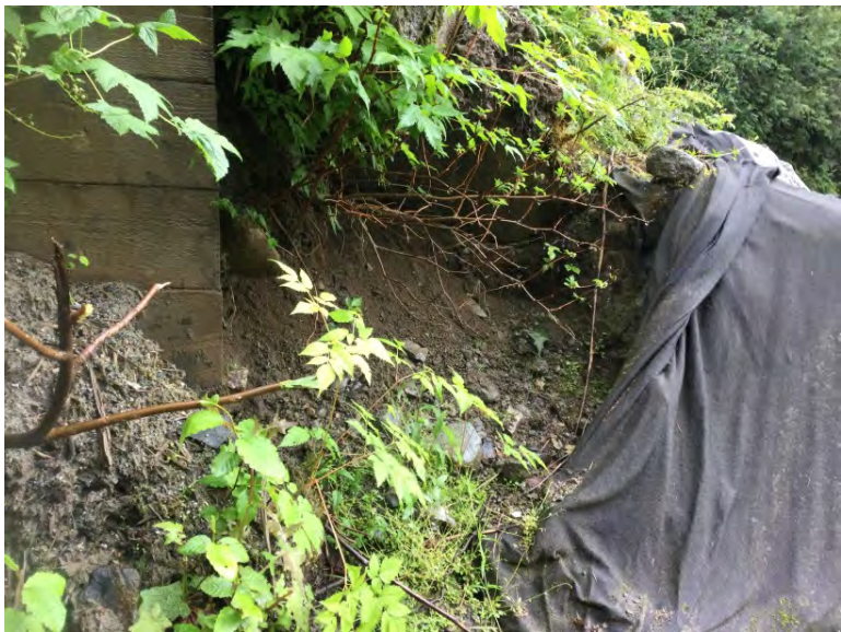
Downstream left bank fill erosion
