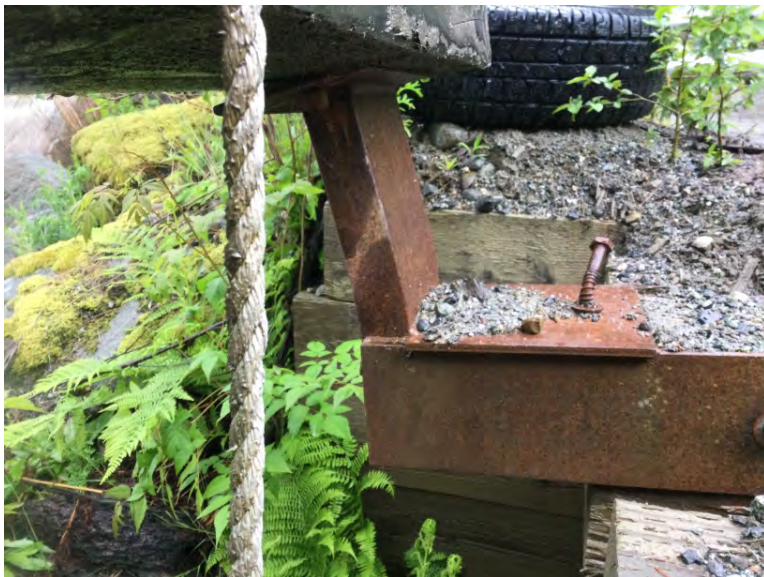
Downstream right bank riser 1 damage
